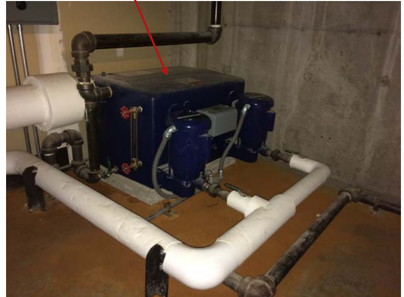
Condensate meter with Duplex pumps
